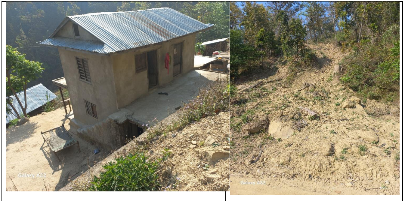
Figure 31: Cracks and displacement observed at the Tilkeni village and debris flow slides at the Sindure Khola road section
