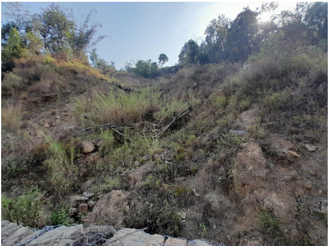
Disturbed bio-engineering structures present in the up slope of the road in crown part of Pokharepata Landslide.
