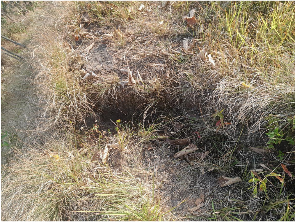
Subsidence and crack seen in the downslope of the road near gully of Hile landslide.
