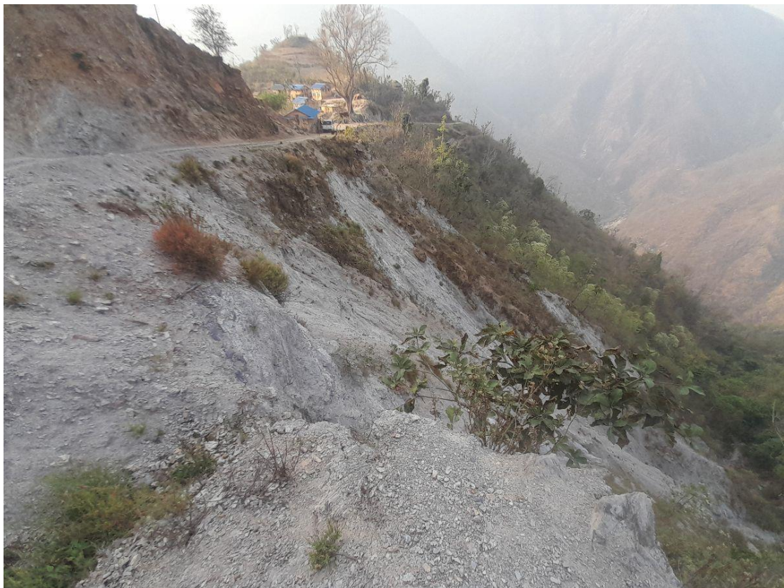
Landslide overview of Lek Kurile landslide.
