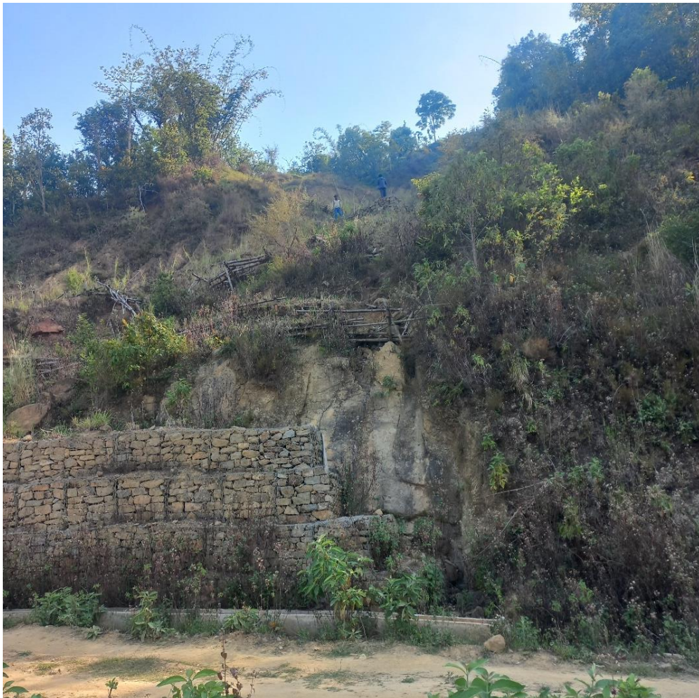
Figure 28: Details view of Pokari Pata landslide
