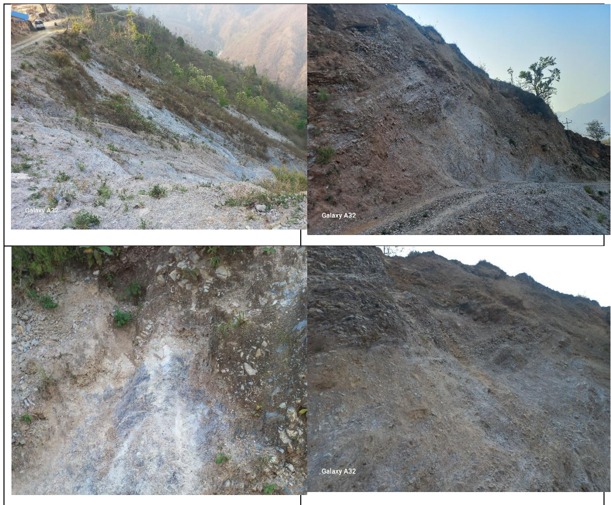
Figure 25: Photographs showing detail view of Lekh Kurule landslides with sheared zone
