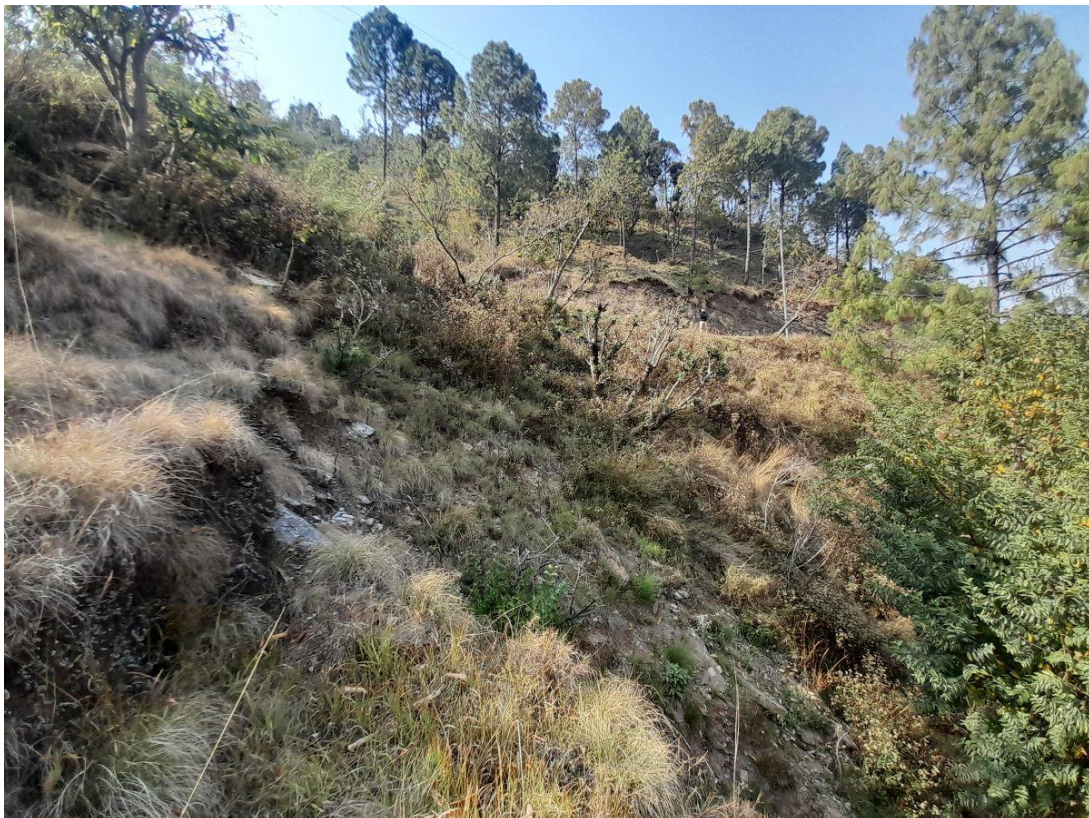
Deformed slope mass in Hile landslide down slope of the road.
